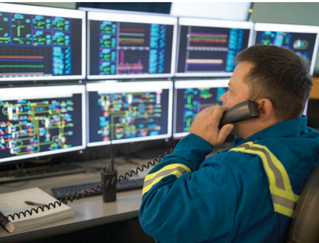
Waterton Control Room
