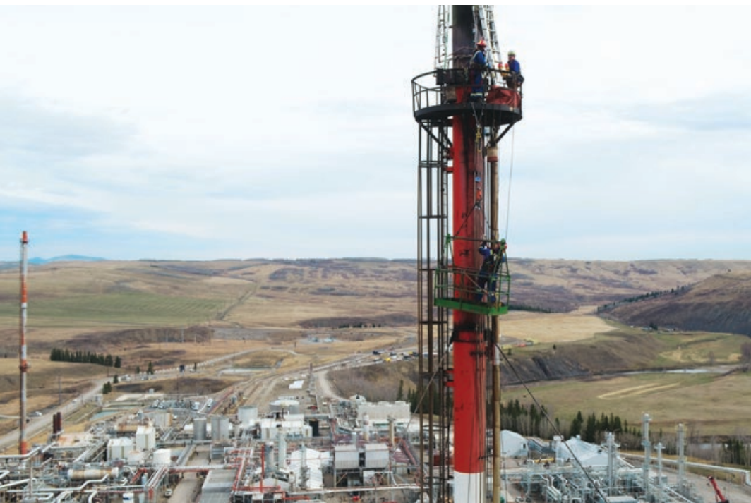
Jumping Pound Facility Turnaround, 2021
